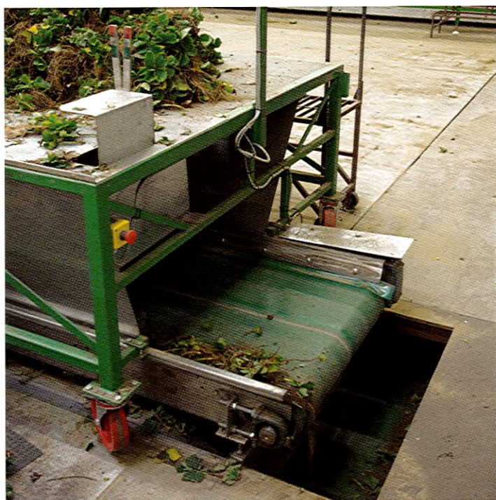
A conveyor belt moves all waste quietly and quickly out of the building.
